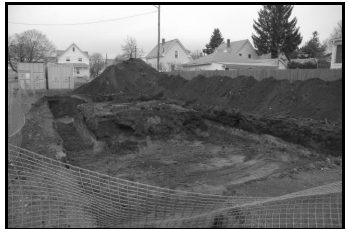
Site is being prepared on Camden Street in Lynn for Habitat volunteers to begin work on June 6 th .
